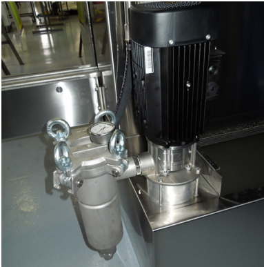
Low Pressure Pump and Filter
